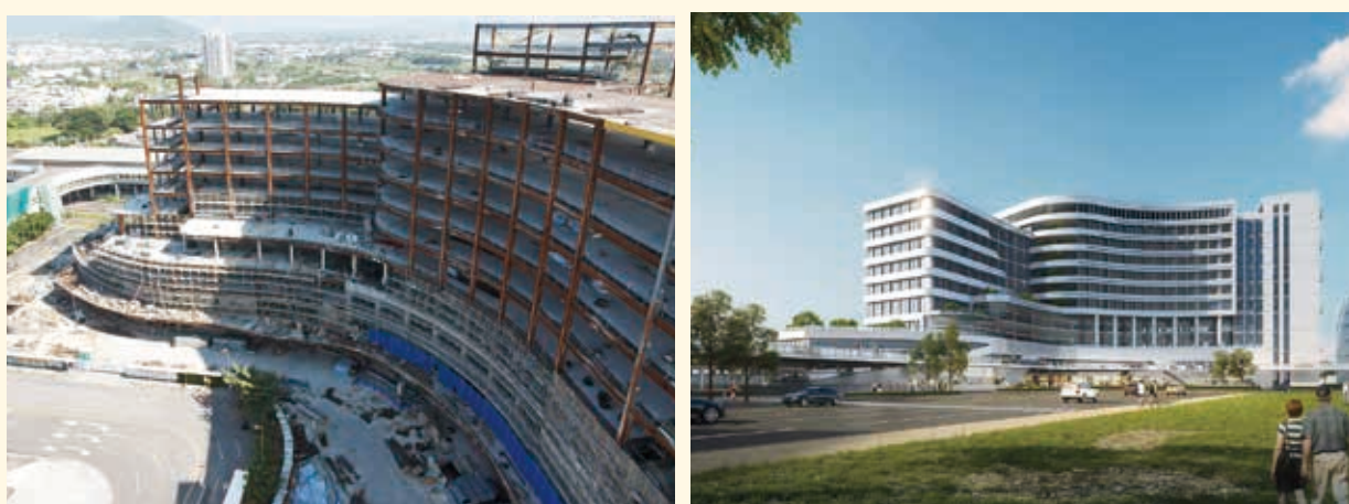
北機廠高醫開發案(興建中) North Depot KMU Development Project (under construction)
