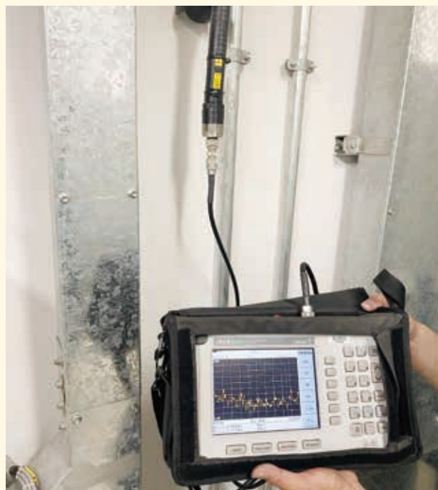
量測訊號傳輸線品質 Measure signal transmission cable quality
