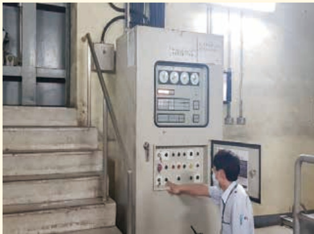
站務人員操作下放隧道防水隔艙閘門 Station staff operating the lower tunnel waterproof compartment gate
