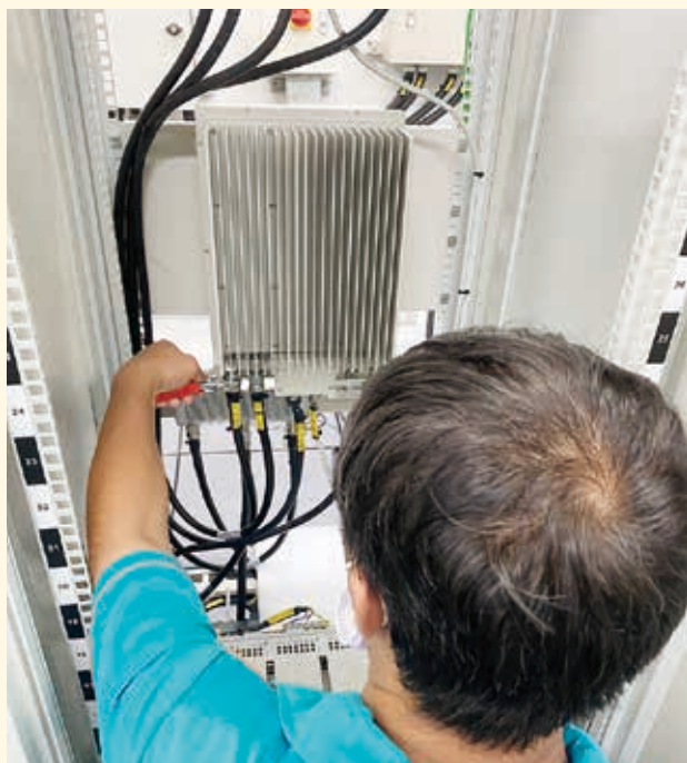
BS422基地台安裝查核 BS422 Base Station Installation Check
