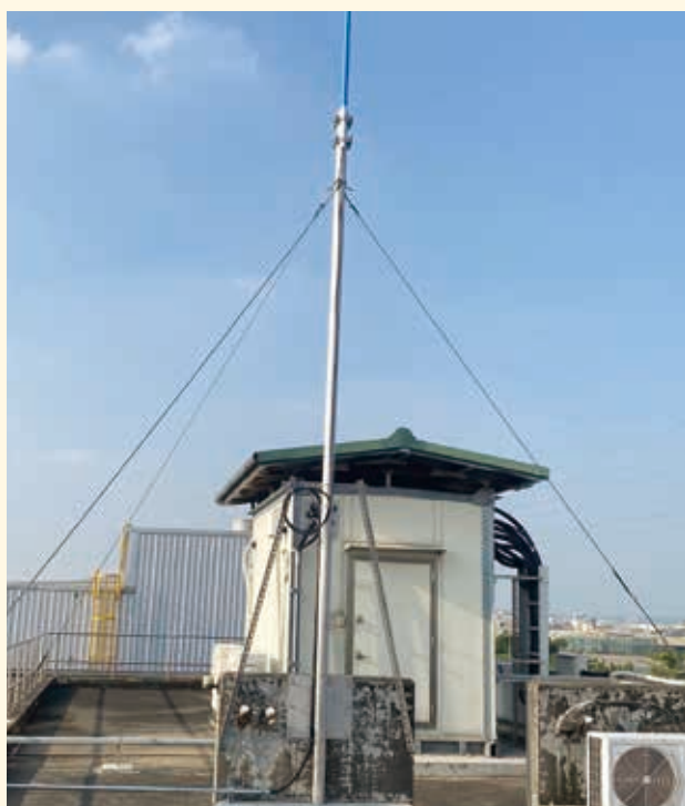
大寮機廠全向性天線安裝完成 Daliao depot omnidirectional antenna installation completed
