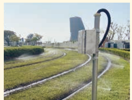
輕軌降噪系統作動 Light Rail Transit Noise Reduction System Activated
